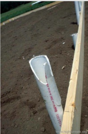
Figure 3. Ground posts damaged during pounding. This can be prevented by pounding on a 2"x4" rather than directly on the PVC pipe.
